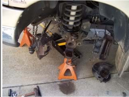
Now its time for the ball joints the upper old is coming out.
